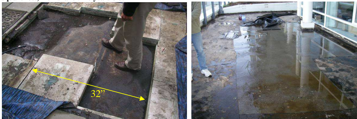
Figure 3: Large "water-bed" type blister lifting pavers Figure 4: Water beneath blistered membrane over entire deck
