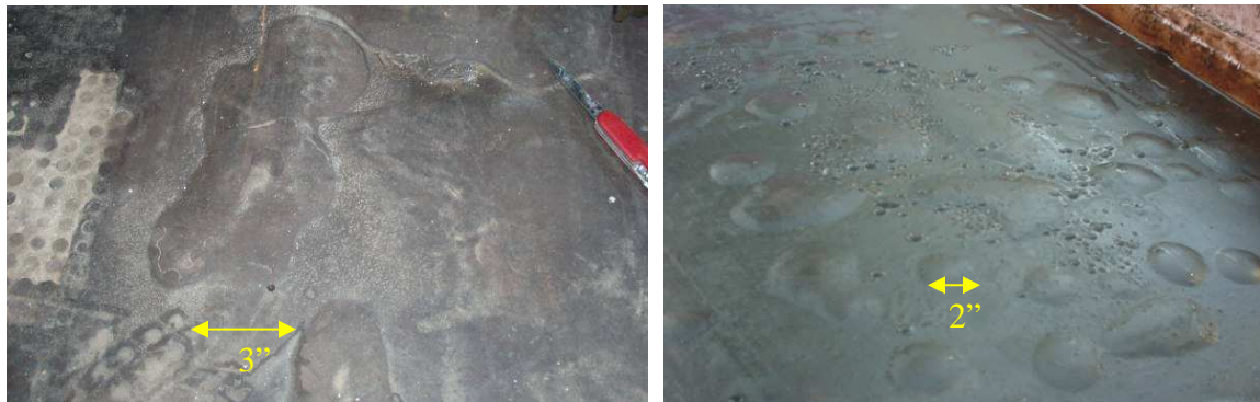
Figure 1 & Figure 2: Typical Blistered Roof Membranes. Blister size ranging from penny sized blisters to areas several square feet, membrane 5-10 years old.
