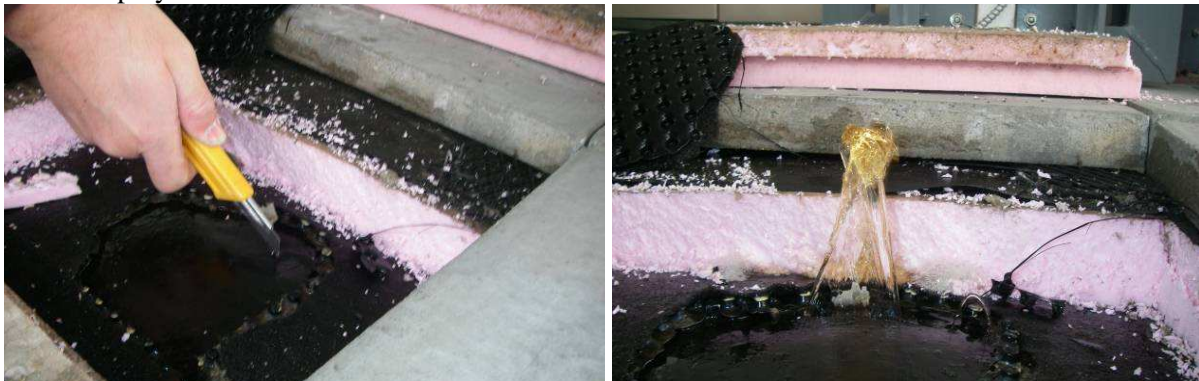
Figure 11 & Figure 12: Cutting of Membrane Blister and expulsion of water during extraction process.
