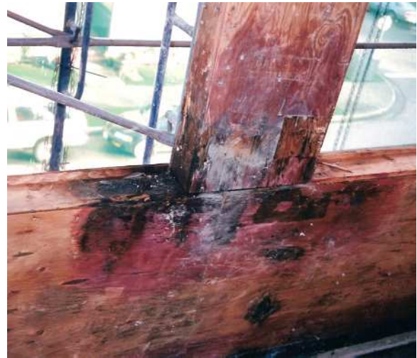
Decay worse under membrane location
