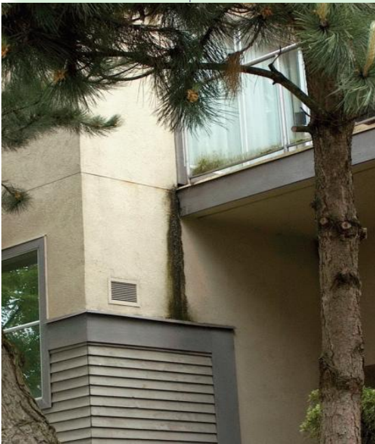
Concentrated balcony runoff leads to an unsightly appearance and potentially premature failure of the wall if not addressed
